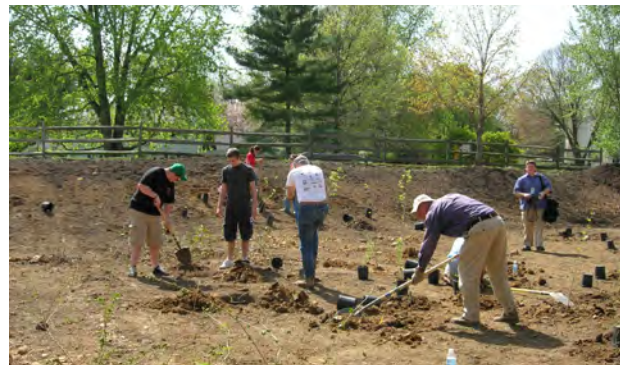
Volunteers planted 300 live stakes and 200 container-grown trees and shrubs. After planting, the basin was seeded with wet and dry native meadow mixes.
